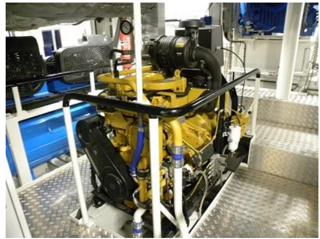
Caterpillar harbour generator set.
