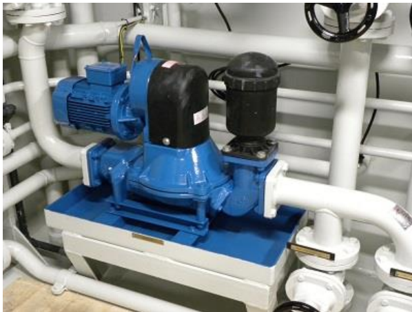
Sewage Pump arrangement
