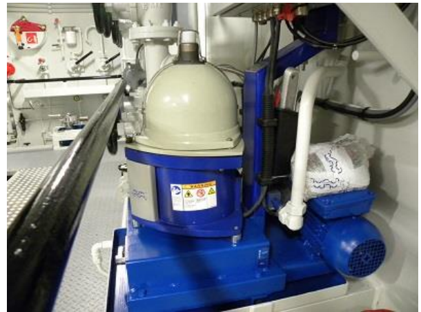
Fuel oil separator
